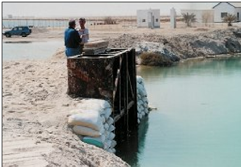
Fig. 7.4 A Water Box Arrangement as used on a Reclamation Project in Bahrain.
